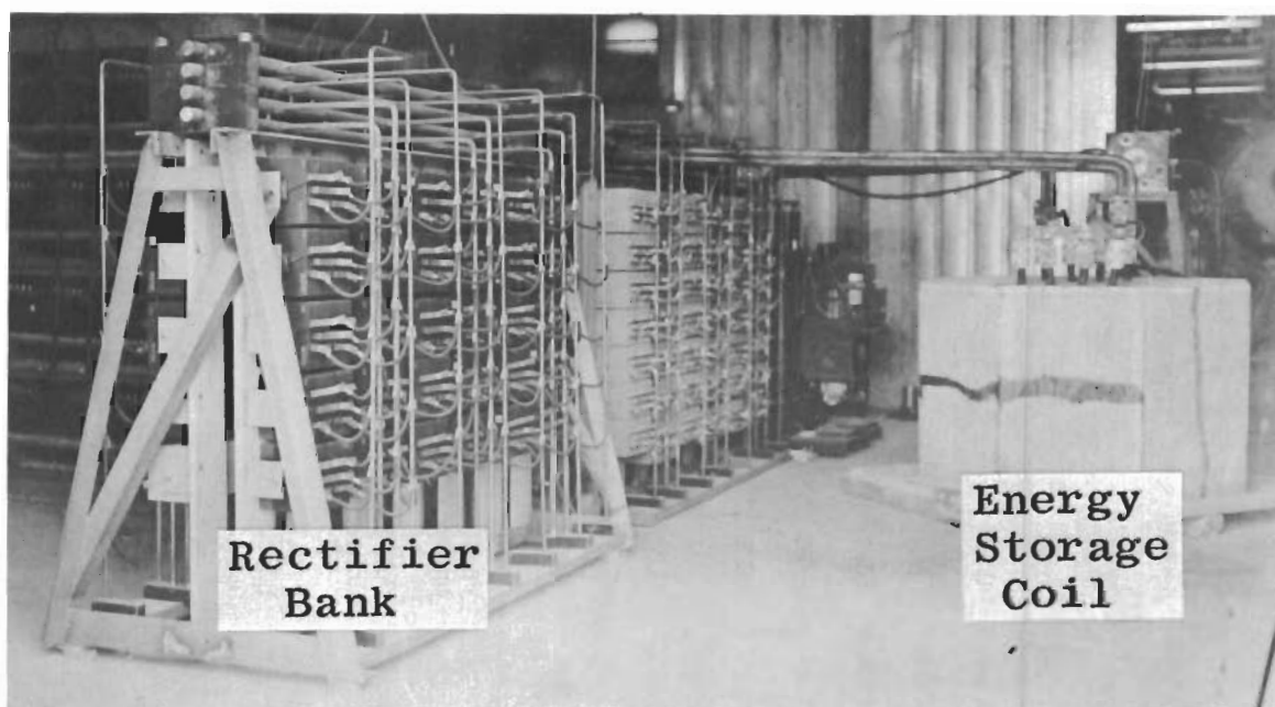
Fig. 20 Selenium Rectifier and Temporary Coil
