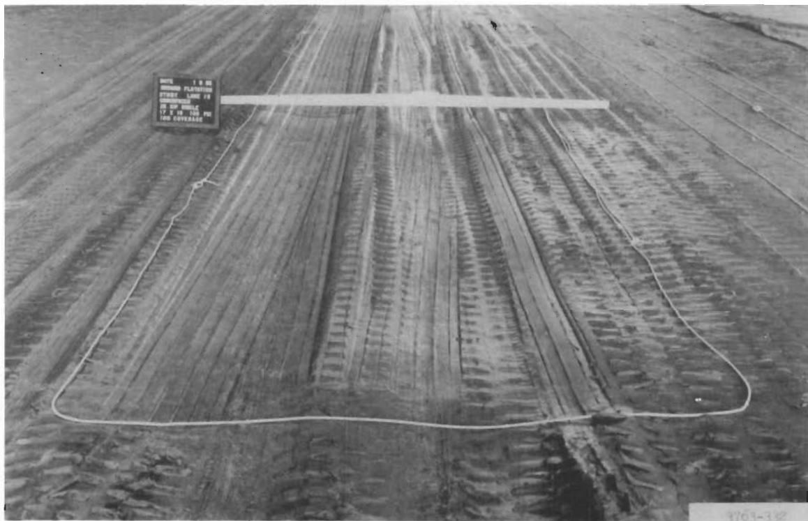
Figure 8. Lane 15; general view showing transverse straightedge measurement at 100 coverages (failure)
