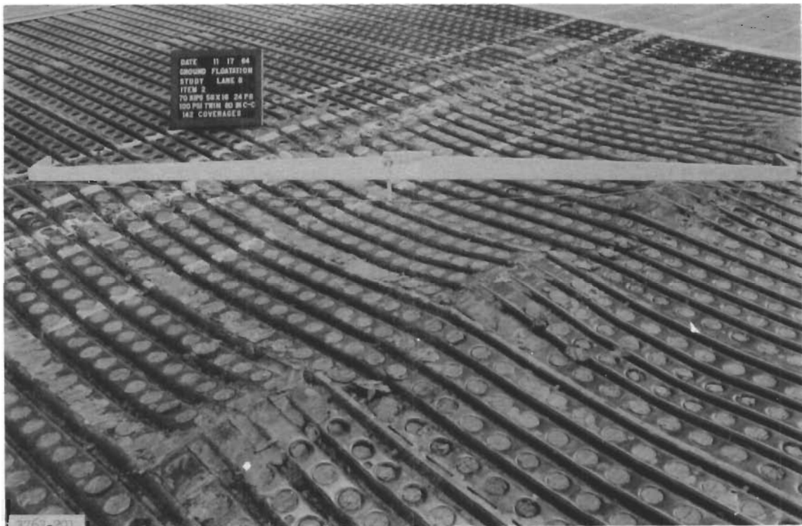
Fig 17. Lane 8, item 2. Diagonal straightedge shows roughness at 142 coverages (failure)
