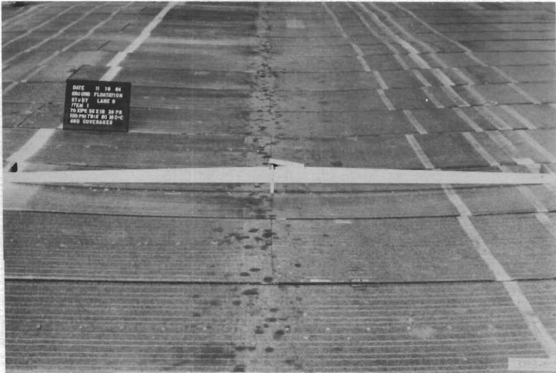
Fig 14. Lane 8, item 1. Transverse straightedge shows roughness at 460 coverages (failure)
