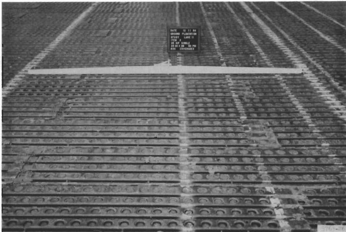
Figure 6. Lane 11, item 2. Transverse straightedge shows slight deformations at 600 coverages
