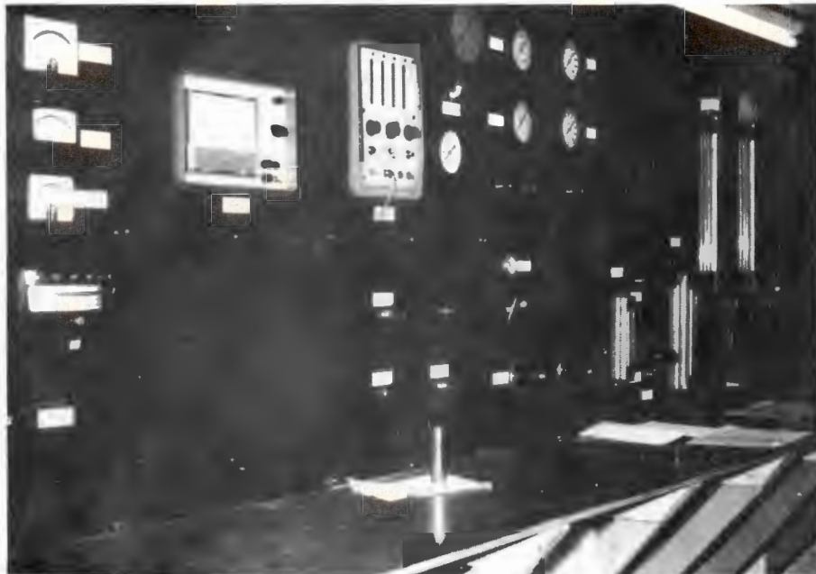
FIGURE 7. INSTRUMENT PANEL - RIG A
