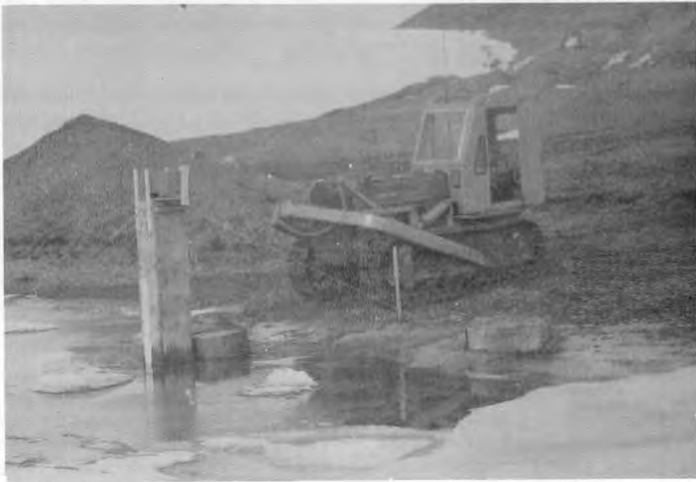
Fig. 3. Tidal gauge stilling well at west end of Ward Hunt Island. The stilling well was anchored by attaching cables from the well to boxes filled with rocks. Total tidal variation was about 18 inches (taken 17 August 1959).
