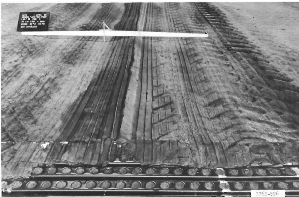
Figure 8. Lane 28, item 3, after 200 coverages of traffic (failure)
