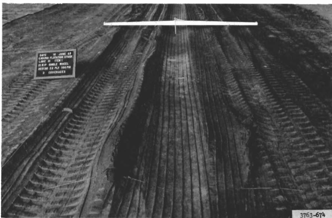
Figure 10. Lane 31, item 1. Transverse straightedge shows roughness at 3 coverages (failure)
