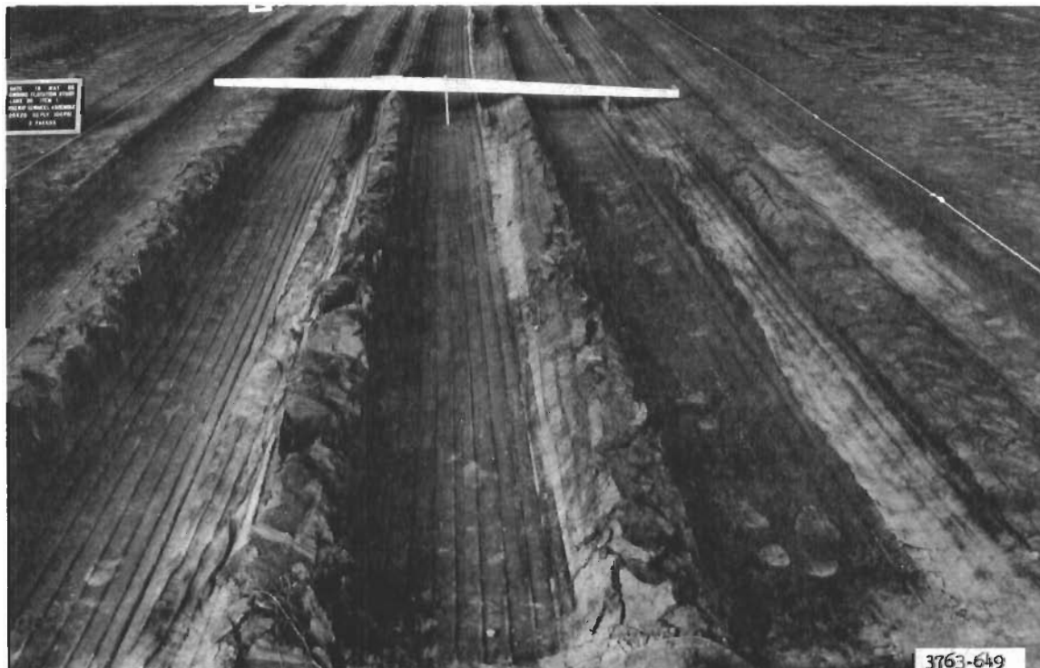
Figure 5. Lane 30, item 1. Transverse straightedge shows rutting at 2.4 coverages (2 passes) (failure)
