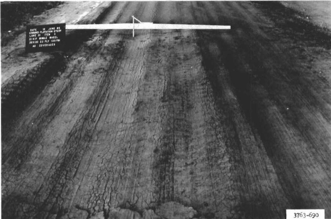
Figure 12. Lane 31, item 3. Transverse straightedge shows roughness at 40 coverages (failure)
