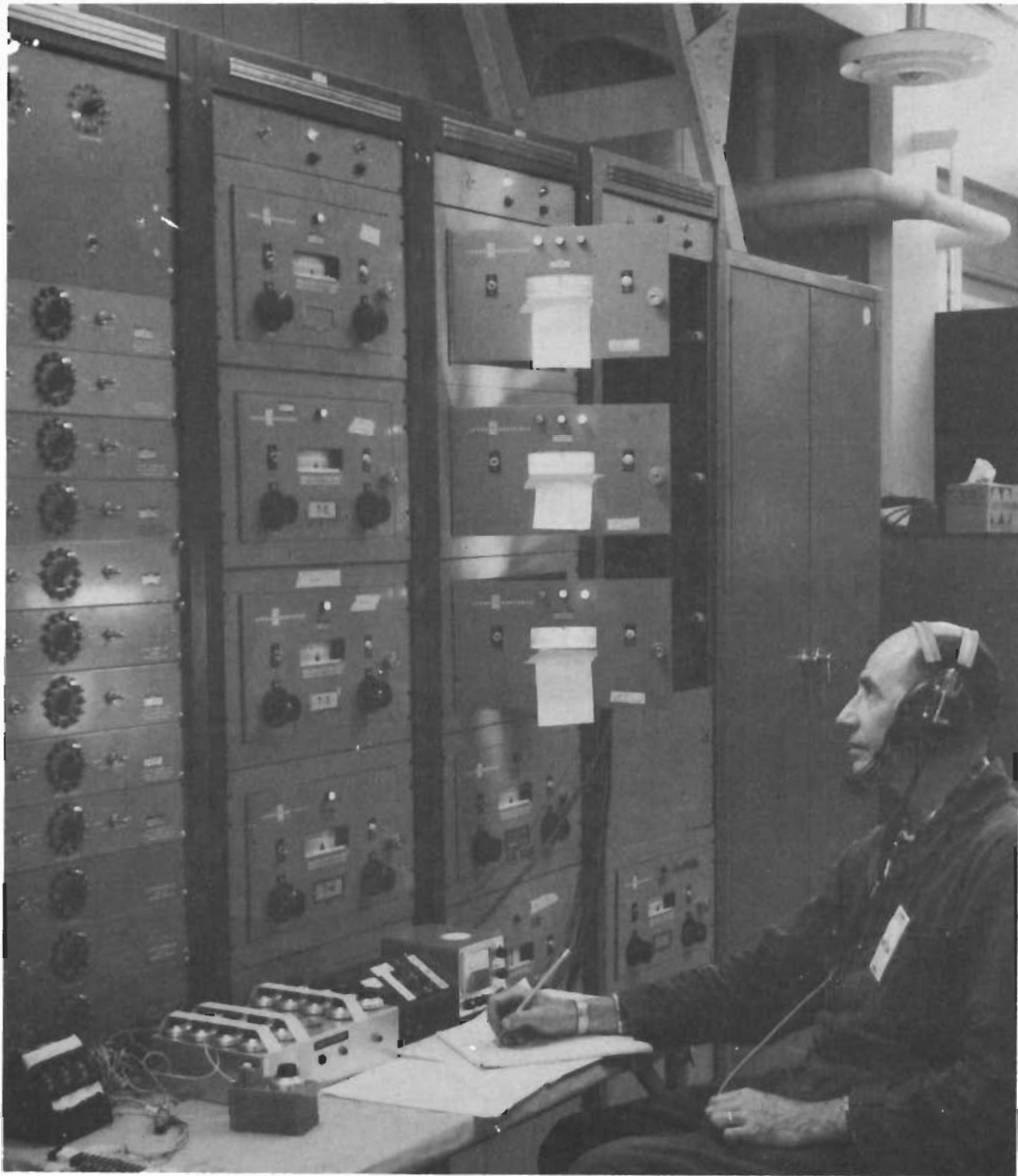
Fig. 6 Photograph of Flap Control and Indicator Panels
