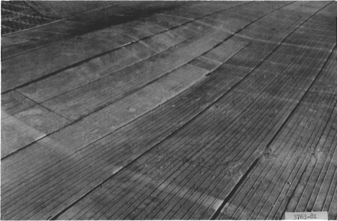
Figure 4. Lane 3, item 1, showing severe localized mat damage at 458 coverages
