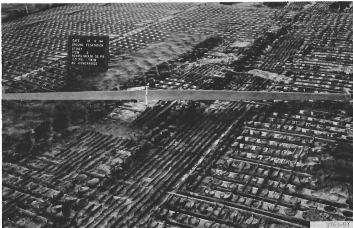
Figure 22. Lane 4, item 2; diagonal straightedge shows roughness at 20 coverages (failure)
