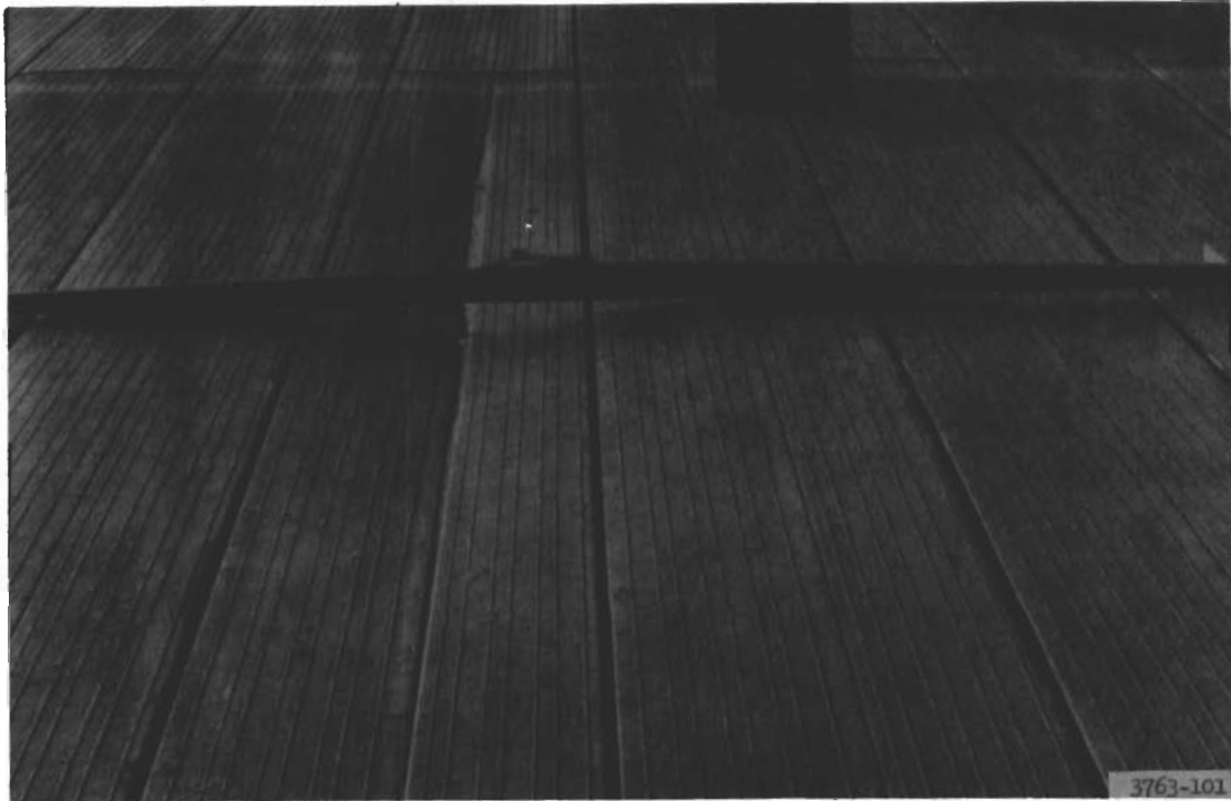
Figure 18. Lane 4, item 1, broken panel in run 15 at 20 coverages (failure)
