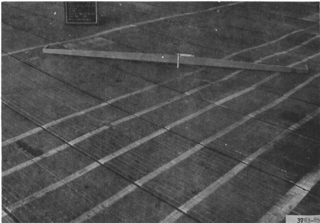
Figure 7. Lane 3, item 1; diagonal straightedge shows roughness at 600 coverages (failure)
