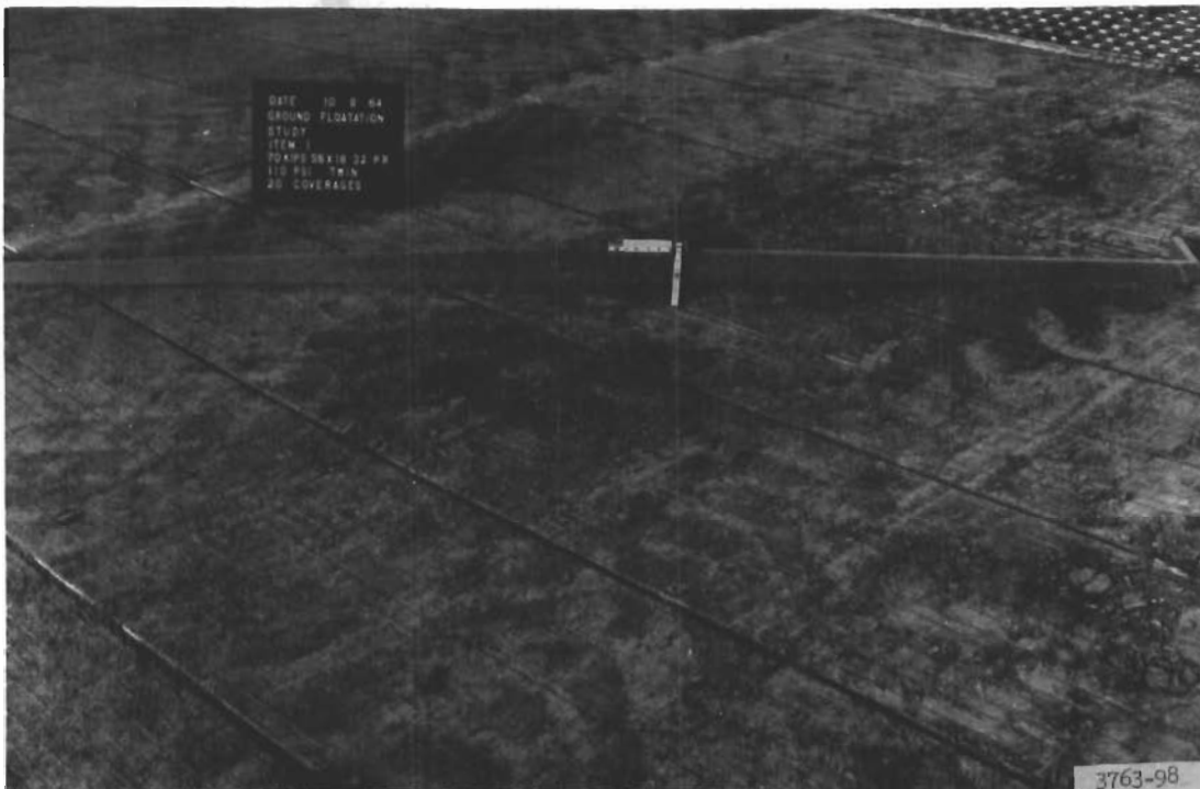
Figure 17. Lane 4, item 1, at 20 coverages (failure)
