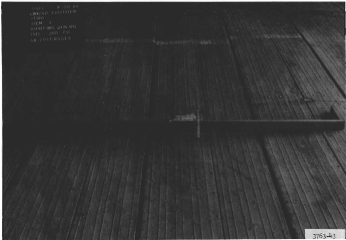
Figure 16. Lane 2, item 3, at 68 coverages (28 postfailure coverages). Longitudinal straightedge shows roughness and mat deformation
